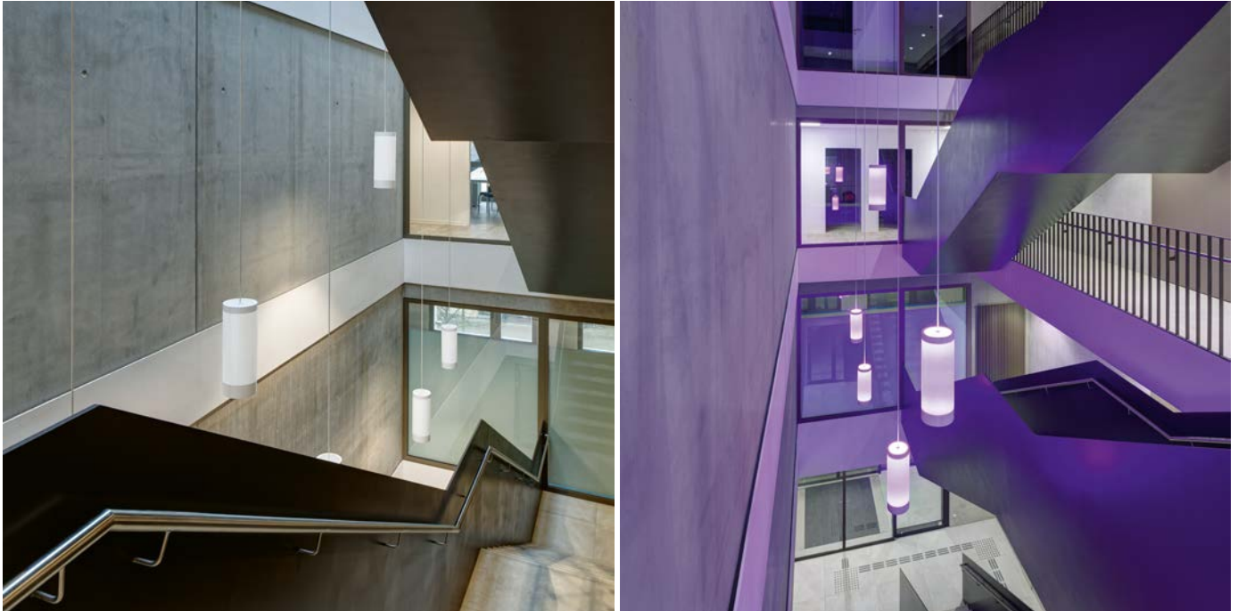
The interplay of architecture and colour-controlled illumination can set accents: For the stairway of a commercial building in Menden that receives heavy public traffic, BEGA pendant luminaire downlights not only provide functional lighting but also surprising entertainment value.
